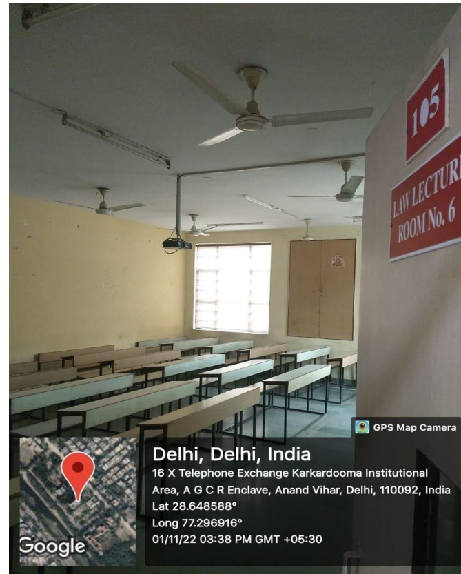
ROOM NO 105,WALL MOUNTED PROJECTOR
