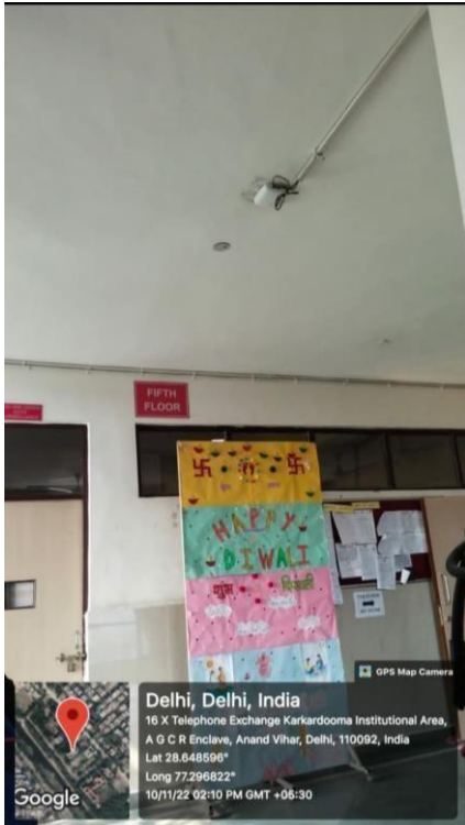
Fifth Floor, Wi-Fi Facility
